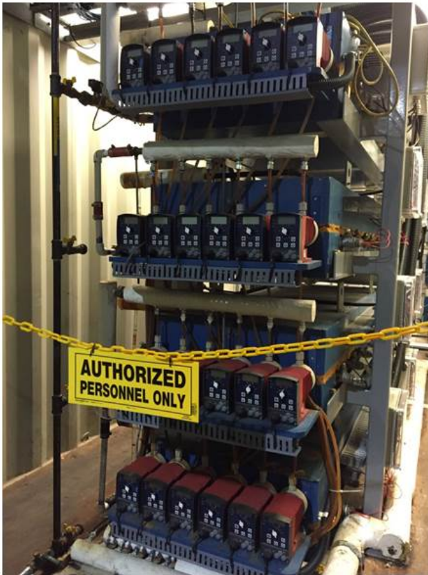
BF Units on west side of red box
